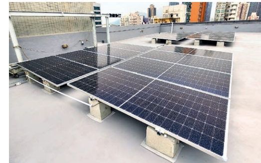
Solar panels at KWP
