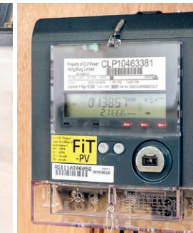
CLP energy meter at SSC
